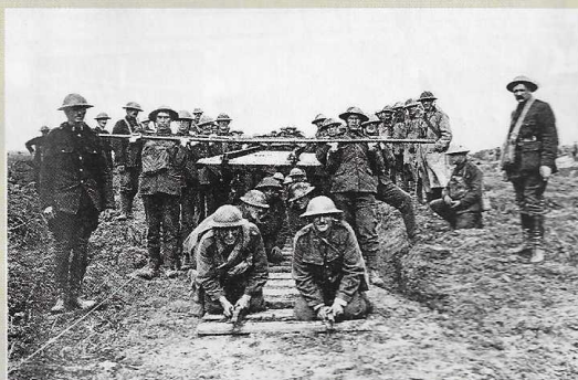
The advantage of 60cm track was that it could be laid quickly with no machinery!
